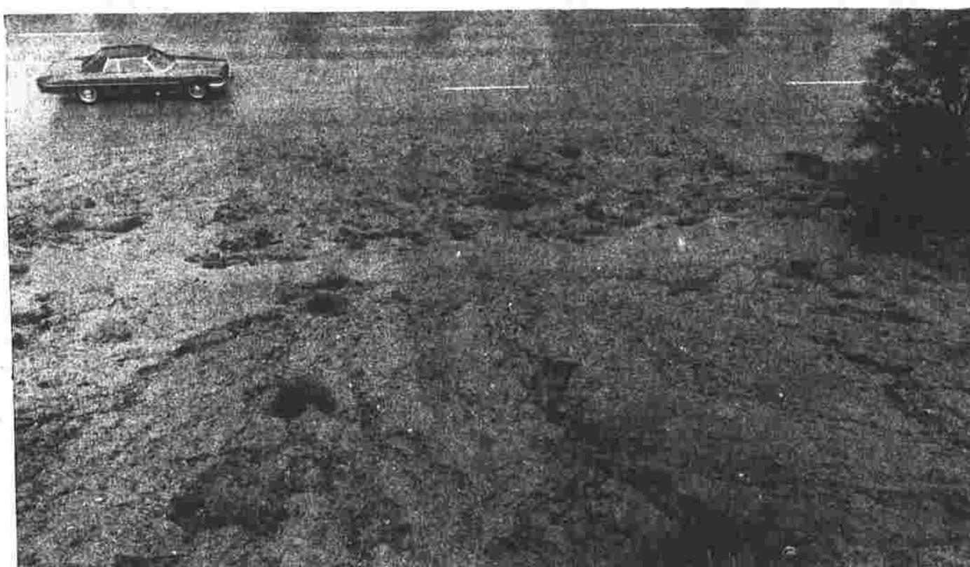
Mud slid down the embankments along Interstate 84 between the Keeney Street and Route 83 exits in Manchester Saturday night, blocking the breakdown lanes.
